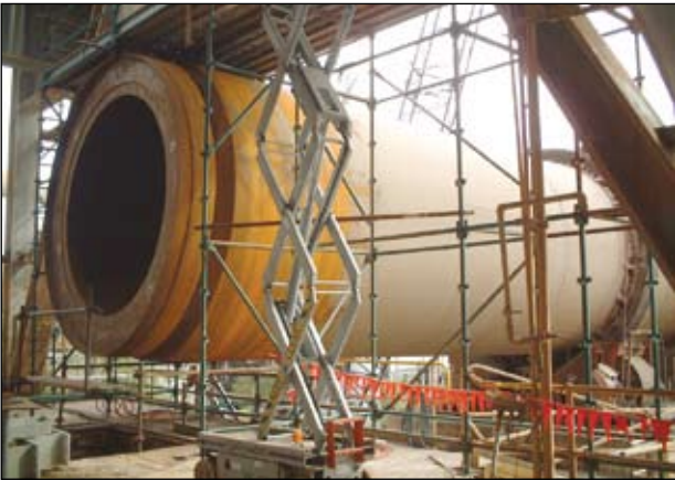
Figure 4. The kiln had a new backend cone and seal ring fitted to suit the Metso preheater.
