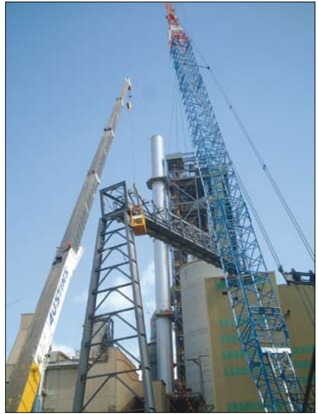
Figure 5. Construction of the limestone conveyor across existing buildings to the lime kiln preheater.
